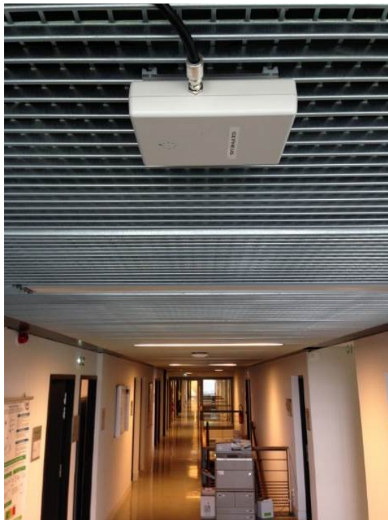
Figure 4.2 – RRU deployed on the ceiling of the corridor.
